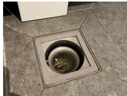
Inlay mounted in drain.
